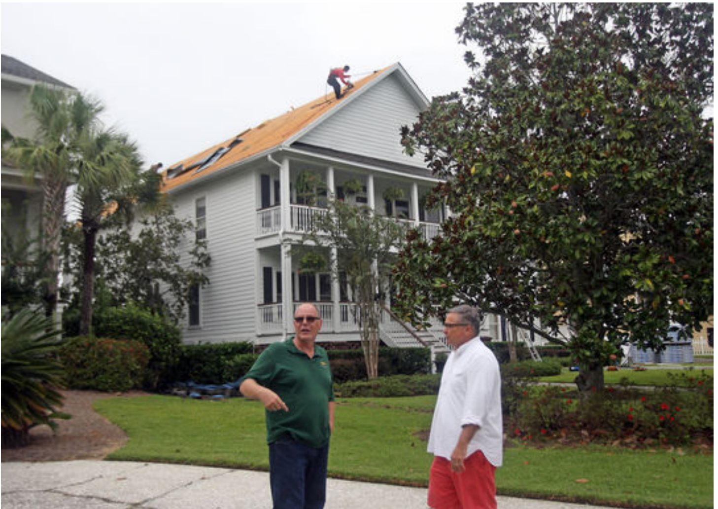
J.R. Yarnall of contracting firm Heritage of Summerville, left, talks with homeowner Jim Terry of Mount Pleasant as workers install a new roof on Terry's Rivertowne community home. Leroy Burnell/Staff
