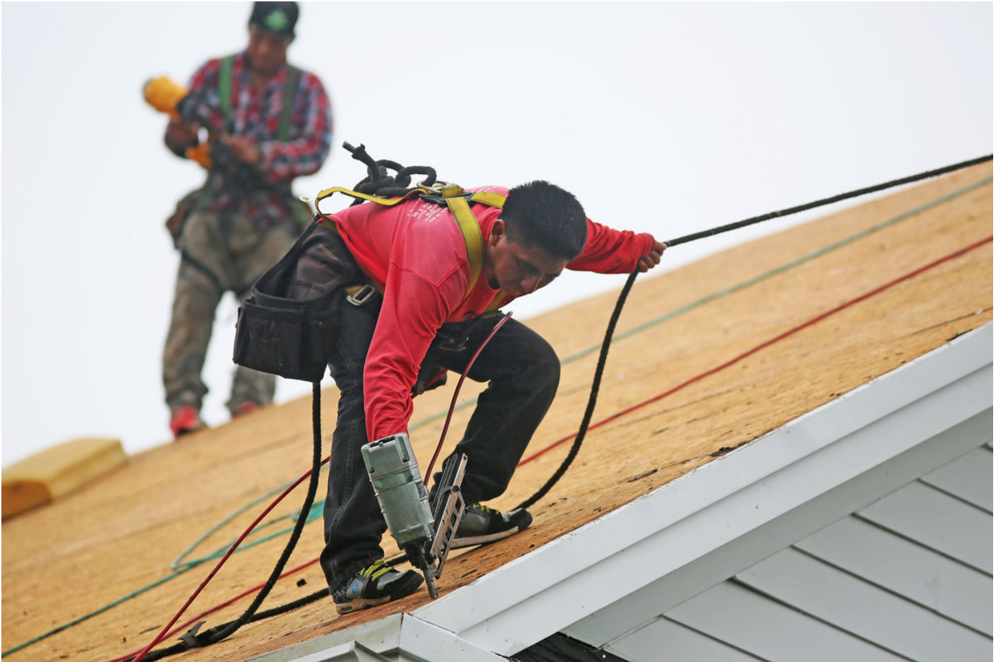
Workers install a new roof last month on the home of Jim Terry in Mount Pleasant. Leroy Burnell/Staff
